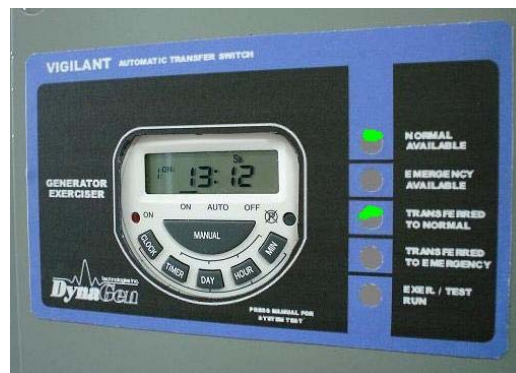
Incorrect LED alignment
