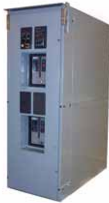
2000 Amperes, 4-Pole, NEMA 1 Enclosed
