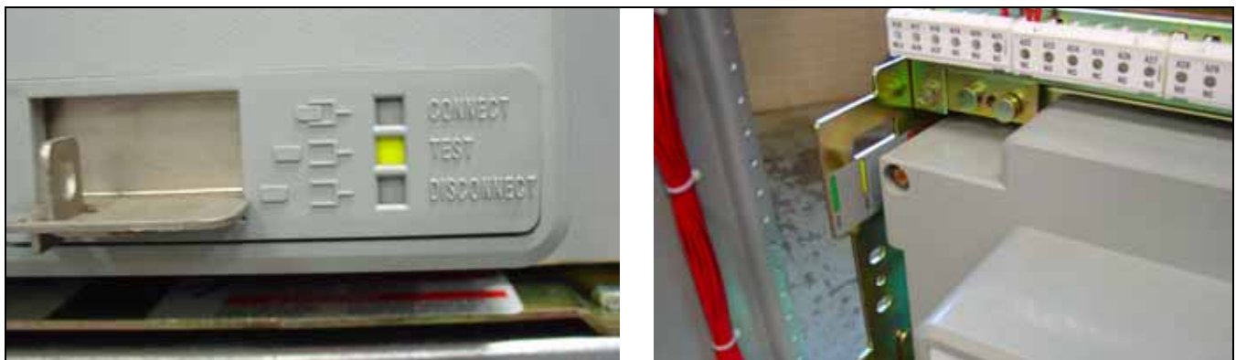
Figure 9. Switching Device in the TEST Position.
