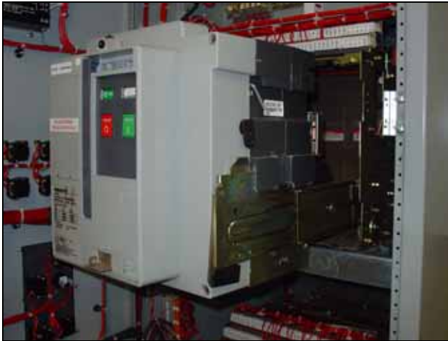
Figure 5. Switching Device Drawn Out from the Transfer Switch.
