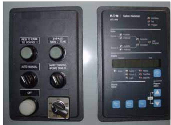
Figure 15. Bypass Isolation Switch.
