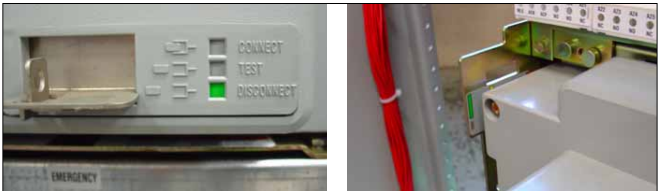
Figure 10. Switching Device in the DISCONNECT Position.
